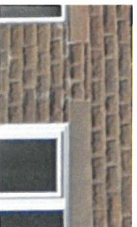
Faux stone with no or plain window details that are poor quality, foreign to the area and out of keeping with the local context.
