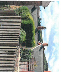
The topography allows close up and direct views of roof tops, features and chimneys.
