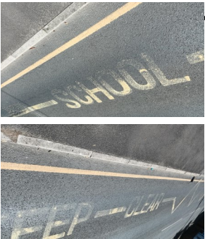
Yellow lines outside the school need re-painting
