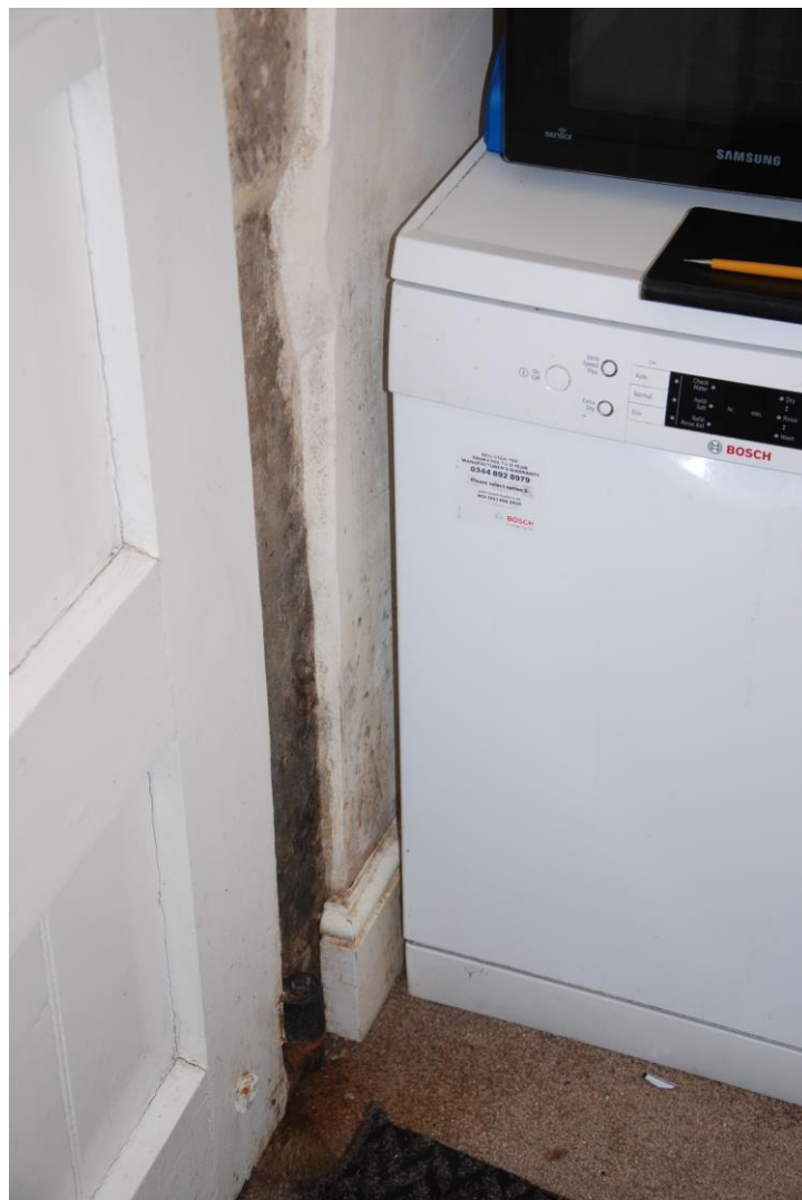
Photo 2: Mould growth adjacent to entrance door
