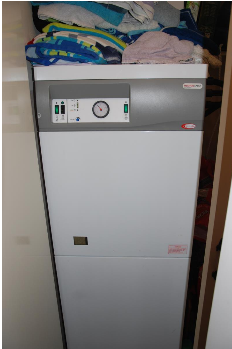
Photo 4: Existing electric boiler
