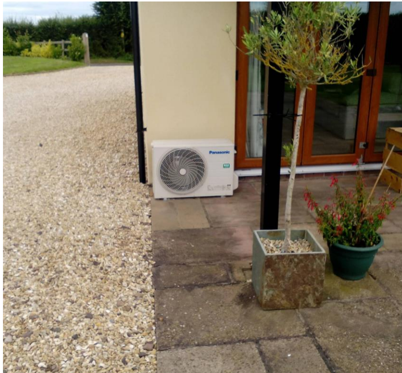
Photo 5: External unit in a residential context
